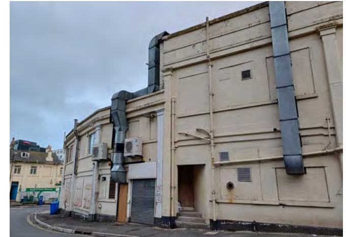
Highly visible plant equipment to structures on the site of the former bus depot detracts significantly from the historic and architectural interest of the conservation area.
