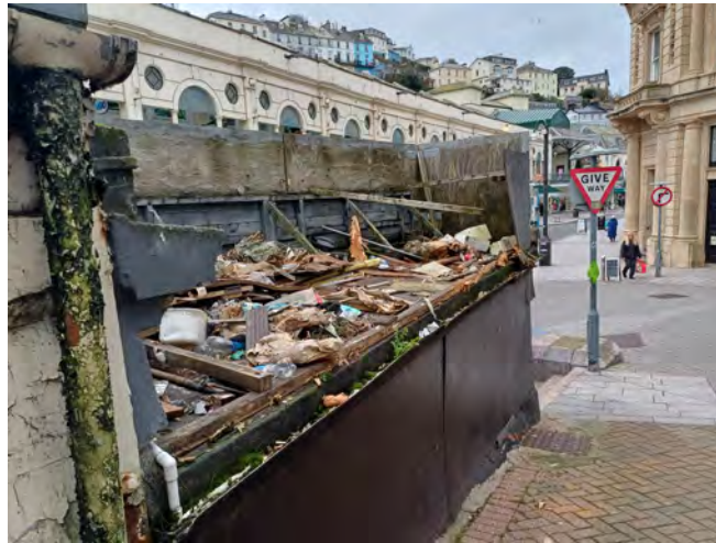
Refuse accruing behind single-storey shops on Fleet Street, at the junction with The Terrace. On the left is a badly deteriorating downpipe.
