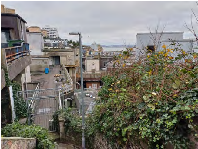
Poor maintenance, including staining, graffiti and overgrown vegetation depreciates the setting of the many listed buildings along The Terrace.
