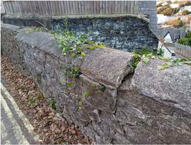
A deteriorating historic boundary wall on Vanehill Road.
