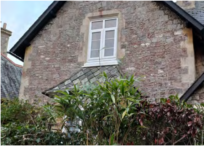
The replacement of the original timber framed windows in this Victorian house on Vanehill Road with uPVC units depreciates the architectural interest of the façade and the wider streetscape.
