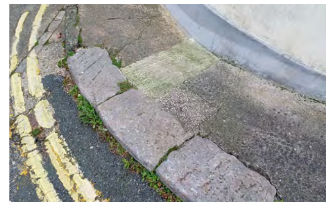
Local limestone and slate can be found in kerbstones across the conservation area.
