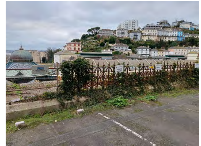
Lack of maintenance to the Grade II listed railings opposite St John's Church on Montpellier Road puts this important asset at risk.
