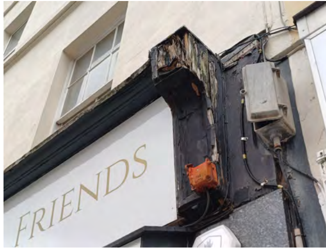
Rotting joinery to a historic shopfront on Fleet Street.
