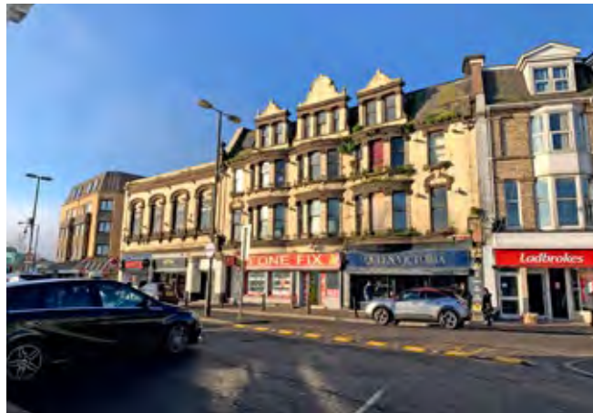
The former Bailey's Hotel on Station Square which is in a poor state of repair on the upper floors. Inoccupation has led to vegetation being allowed to grow on the front façade, windows become missing, and rainwater goods left to fail causing the building to be in a derelict condition.
