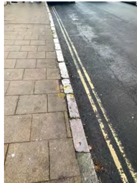
Surviving historic kerbstones on Palace Avenue, with replacement modern slabs to the pavement and tarmacked road.
