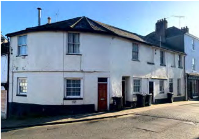
A listed house on the corner of Winner Street and Church Street which has been externally painted in a modern non-permeable paint leading to areas of cracking, bubbling and failure. The timber windows are also rotting in places.
