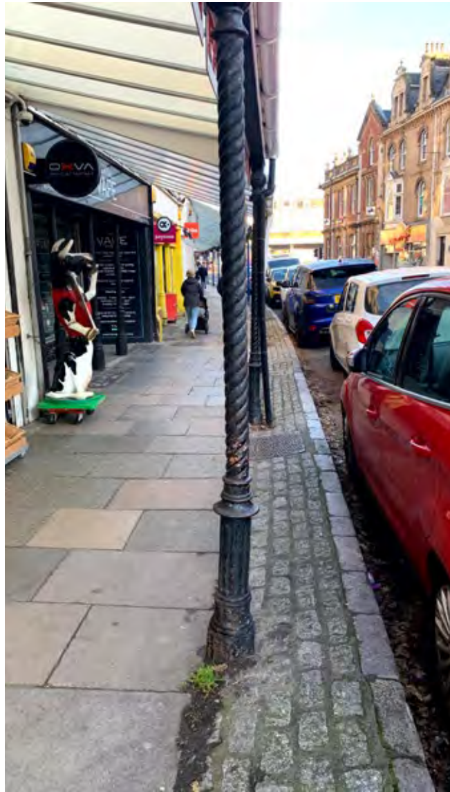
The cast iron columns of the former department store on Palace Avenue.
