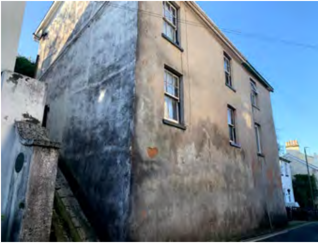
A house on Winner Street which has been externally rendered in concrete, leading to significant issues with dame which is causing areas of the render to fail.
