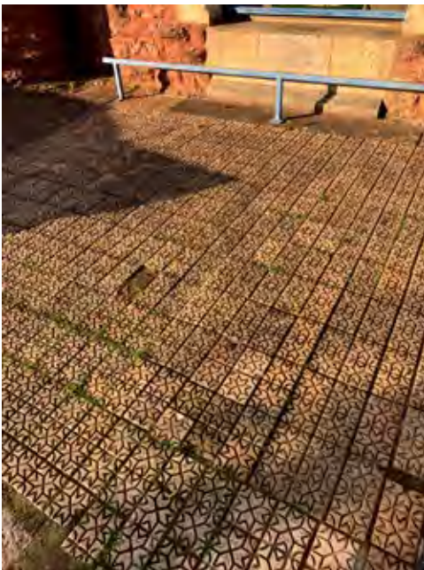
The cream pavers in situ in the forecourt of the Palace Avenue Methodist Church.
