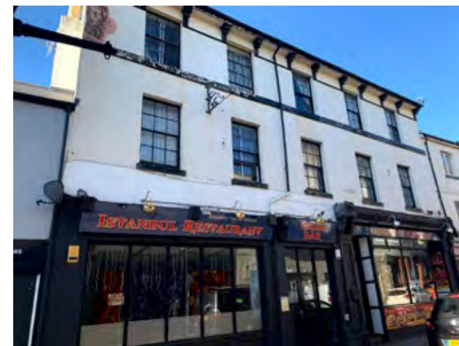
A historic shop on Winner Street which has deteriorating fabric on the upper floors, including areas of failed render and rotting timberwork including windows.
