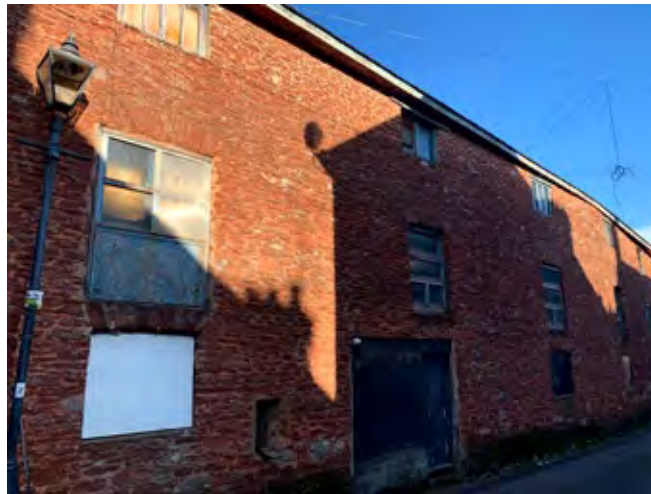
A former listed warehouse on Kirkham Street, later used as a mechanics garage and now unoccupied.
