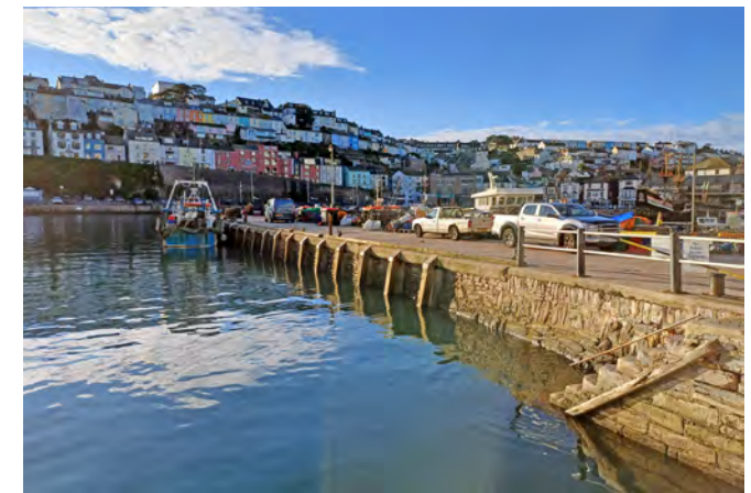
Eastern Quay at Brixham Harbour, in situ by 1781 and still in use today.
