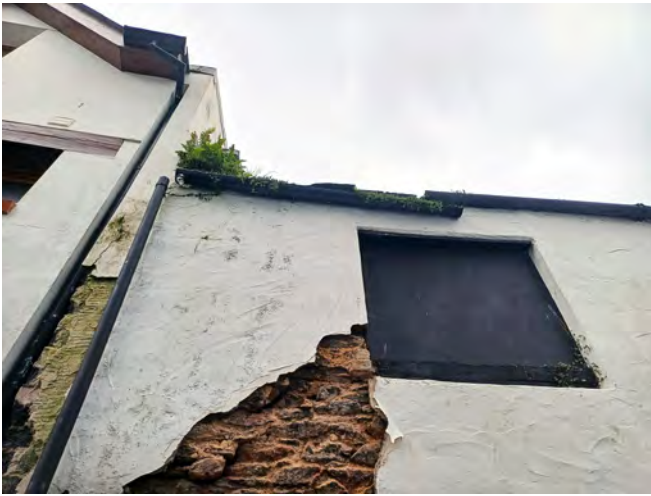
An example of a blocked and broken gutter and failing render to a property on Pump Street.
