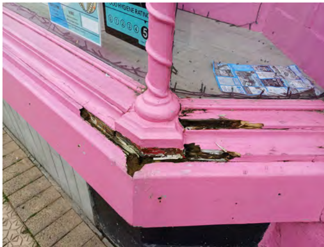
Rotting timber detracts from the aesthetic impact of this traditionally styled shopfront on Fore Street.
